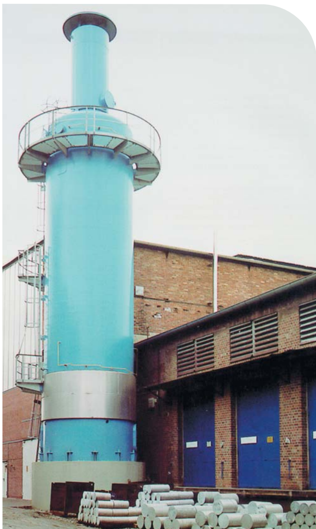
Absorption column of the airwash system.
